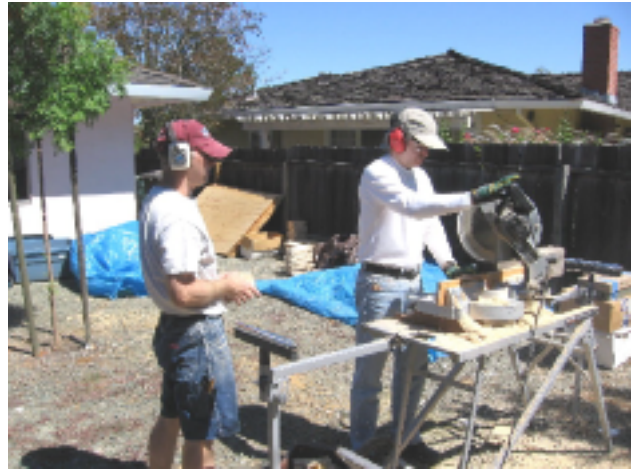
A miter (or chop) saw can cut the angles for the sides, trim the corners of the bottoms, and cut the bevels on the roof pieces.
